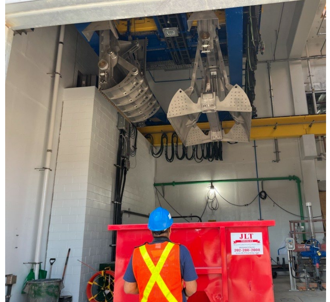
Rake and clamshell system testing ahead of recent wet weather events. A roll off dumpster has been placed in the screening room to collect removed debris.
