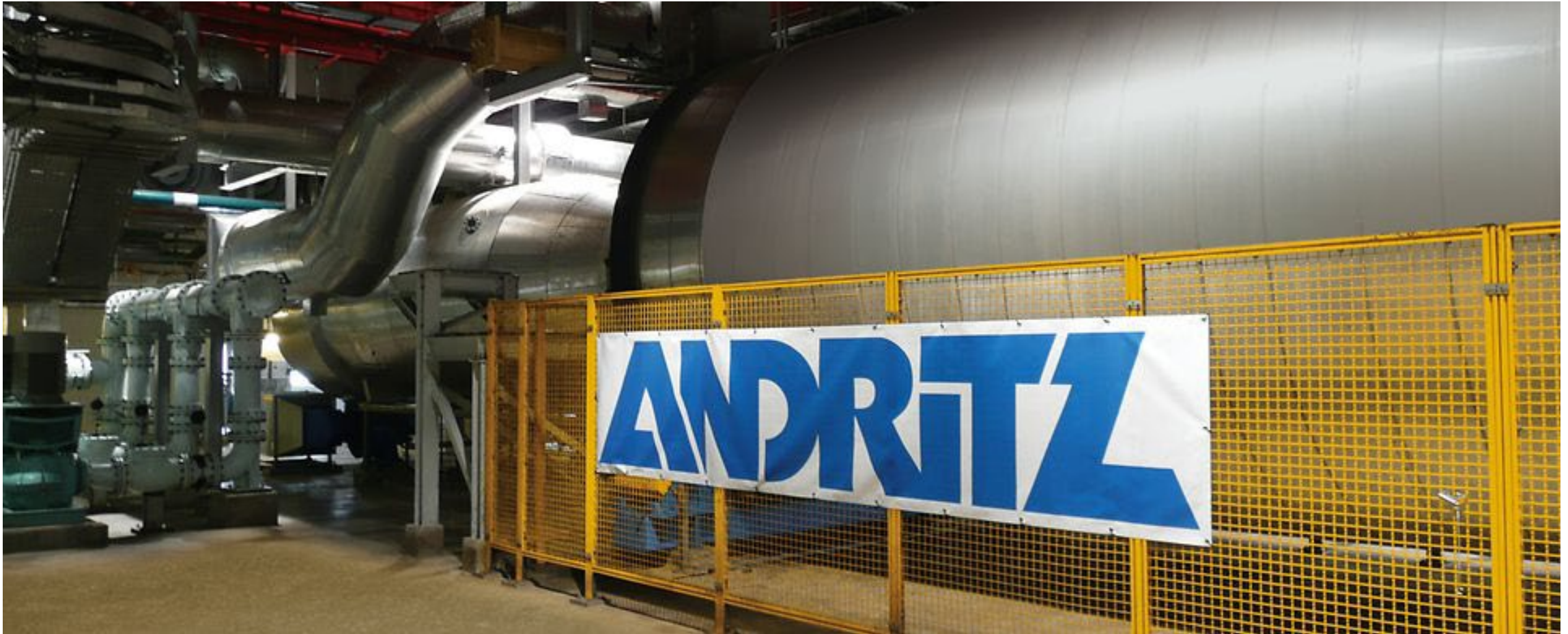
World's largest municipal sludge drying plant in Changi, Singapore. Photo credit: Andritz
