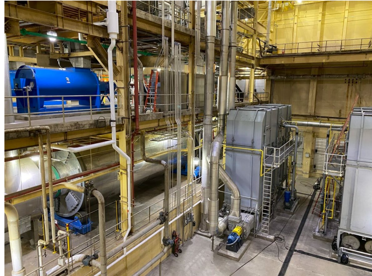
Louisville, KY thermal drying facility for biosolids
