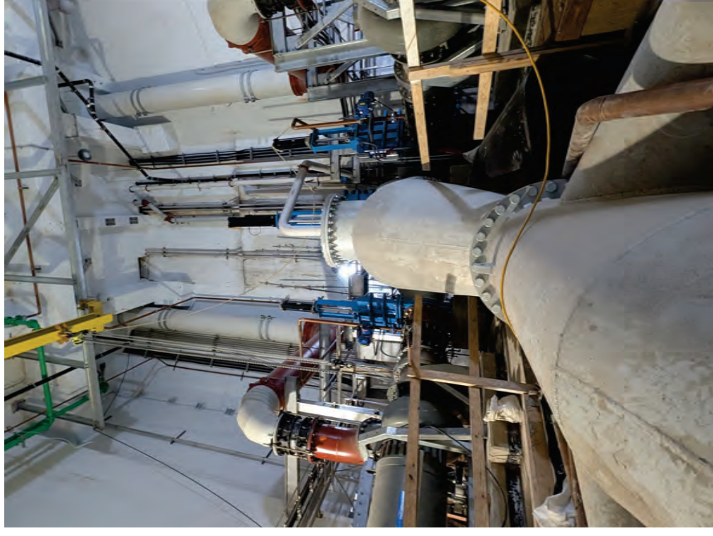
Tunnel Dewatering Pumping Station – READY FOR FLOW
