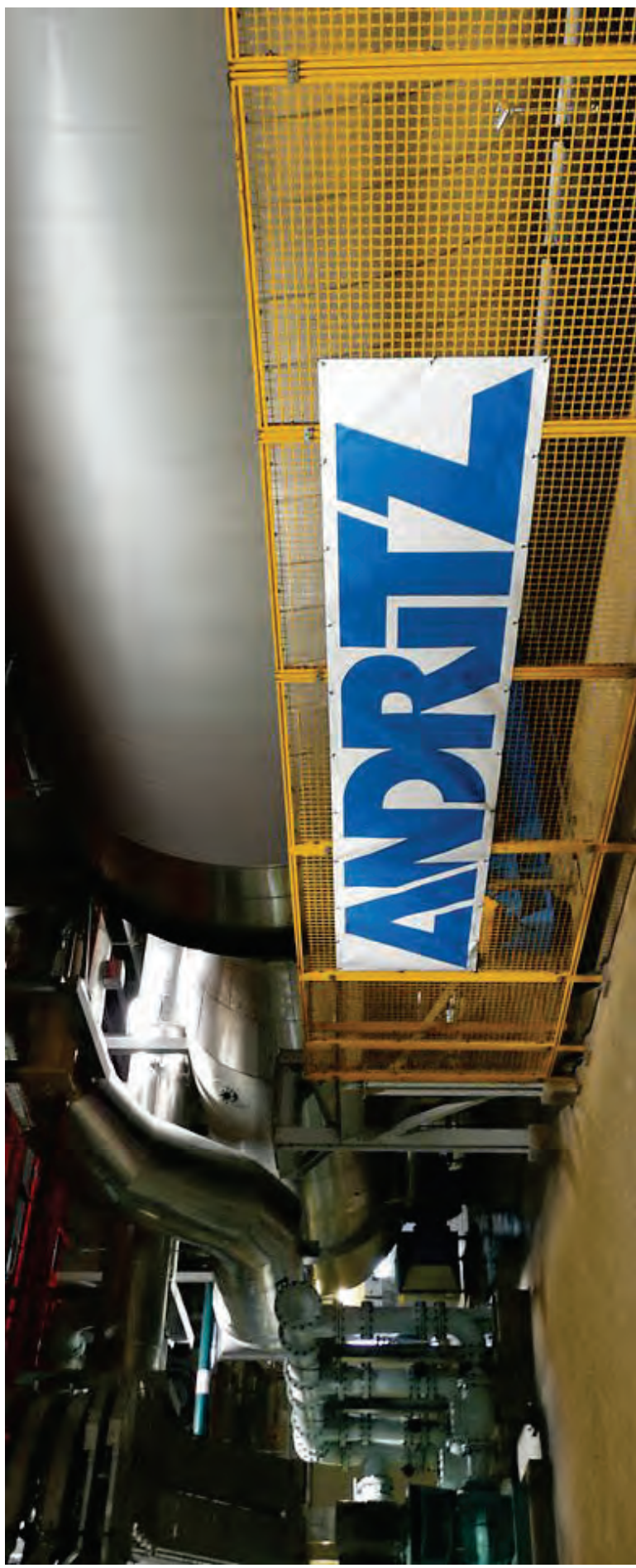
World's largest municipal sludge drying plant in Changi, Singapore. Photo credit: Andritz
