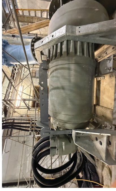
Tunnel dewatering pumping system is READY FOR FLOW!
