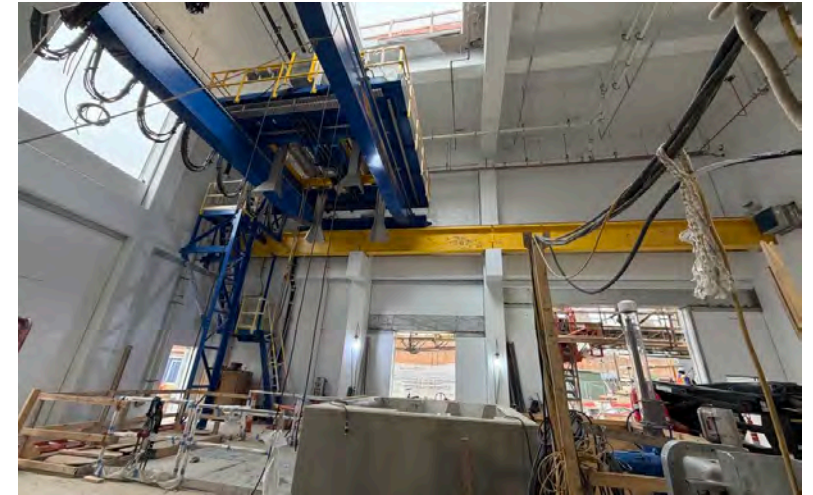
Screen room with overhead clam and rake system
