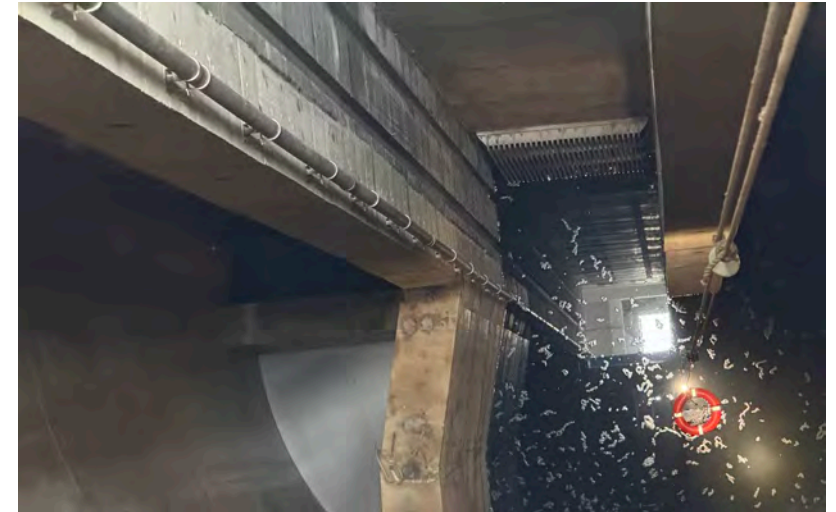
View looking down into the flooded screening shaft
