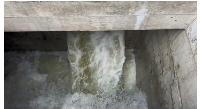
Three pumps operating simultaneously at full speed circulated approximately 120 MGD of flow
