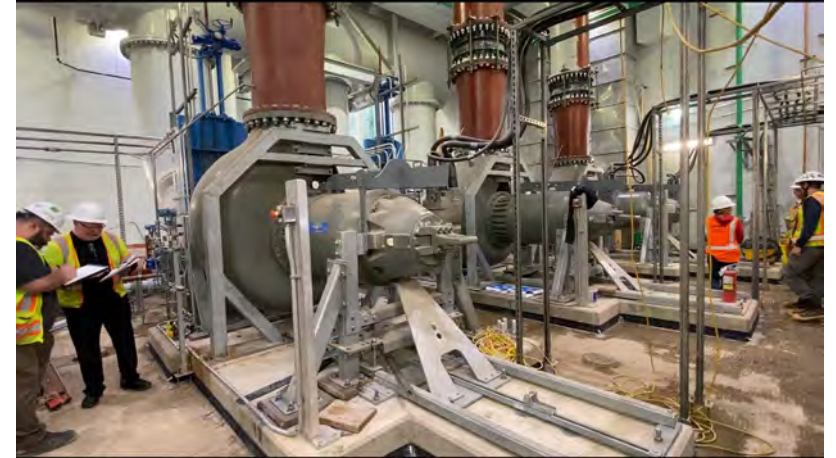
Wet Weather Pumps were operated independently and simultaneously
