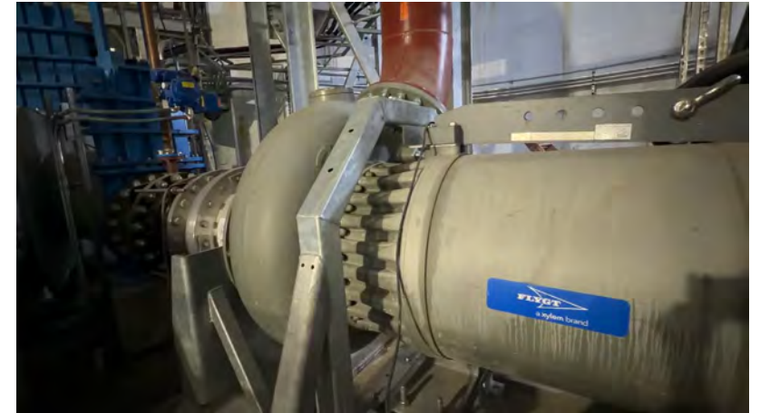
Functional Testing of Tunnel Dewatering Pump #2 (20 MGD)
