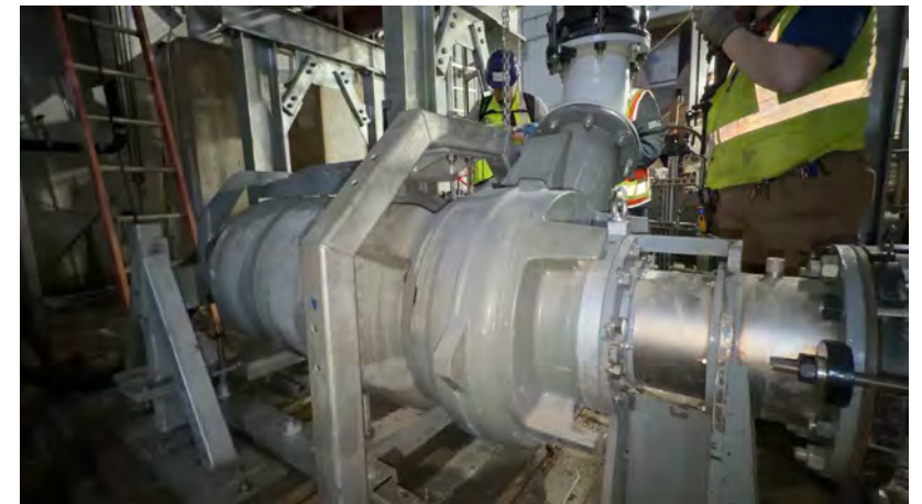
Functional Testing of Solids Handling Pump #2 (5 MGD)
