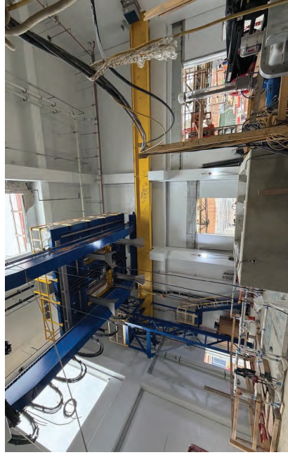
Screen room with overhead clam and rake system
