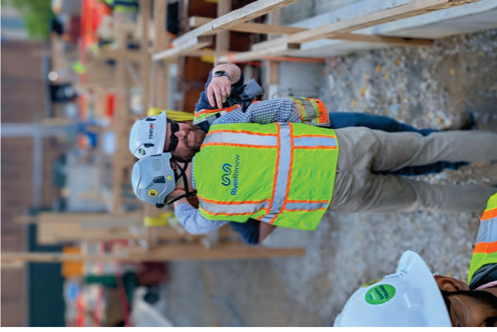
The team celebrates the commissioning of Tunnel Dewatering Pump #1 on April 30, 2026
