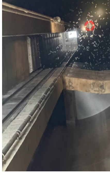
View looking down into the flooded screening shaft
