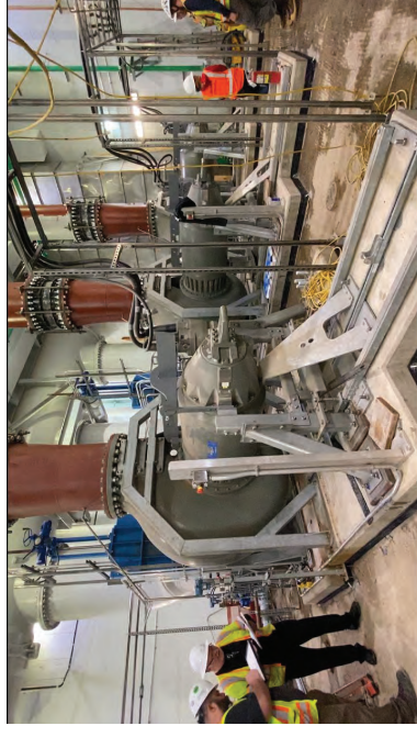
Wet Weather Pumps were operated independently and simultaneously
