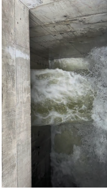
Three pumps operating simultaneously at full speed circulated approximately 120 MGD of flow
