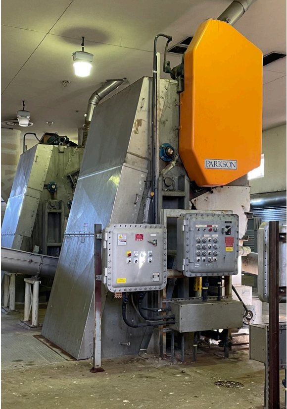
Upgrade two (2) fine screens
