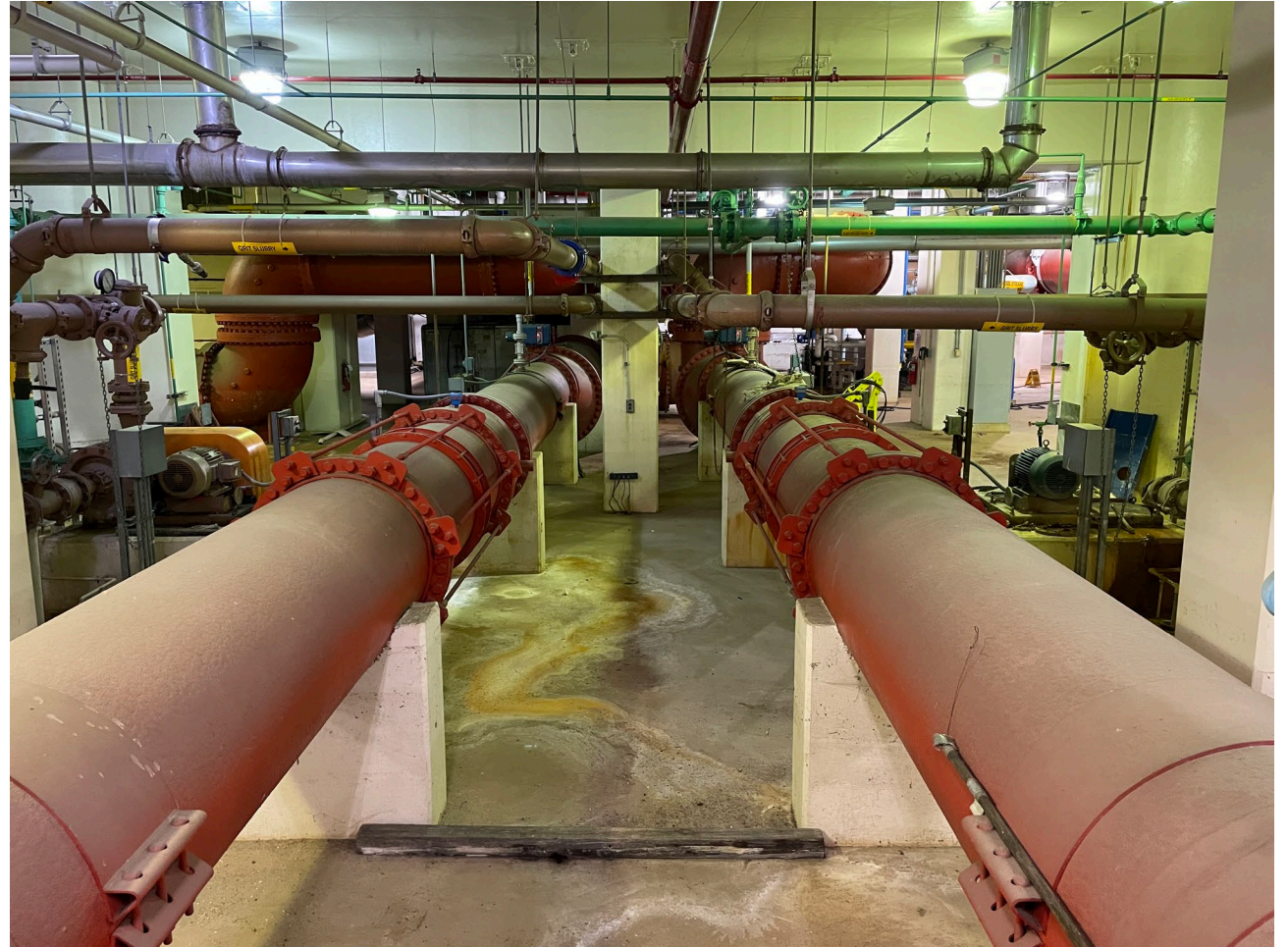
AlexRenew's Primary Influent Conduits in Building K
