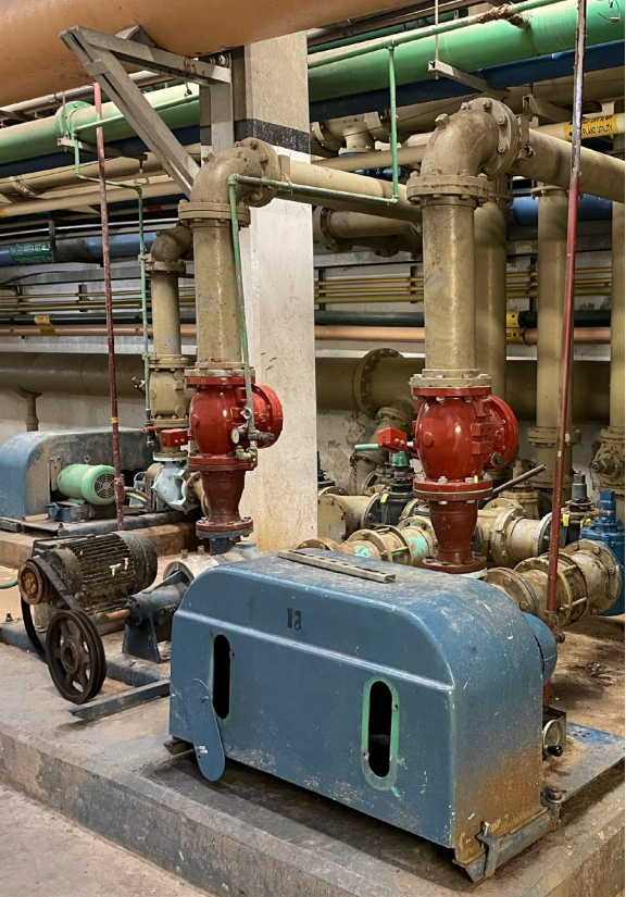
Replace twelve (12) primary sludge pumps
