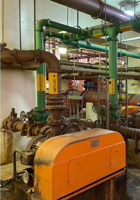
Replace two (2) vortex grit separators
