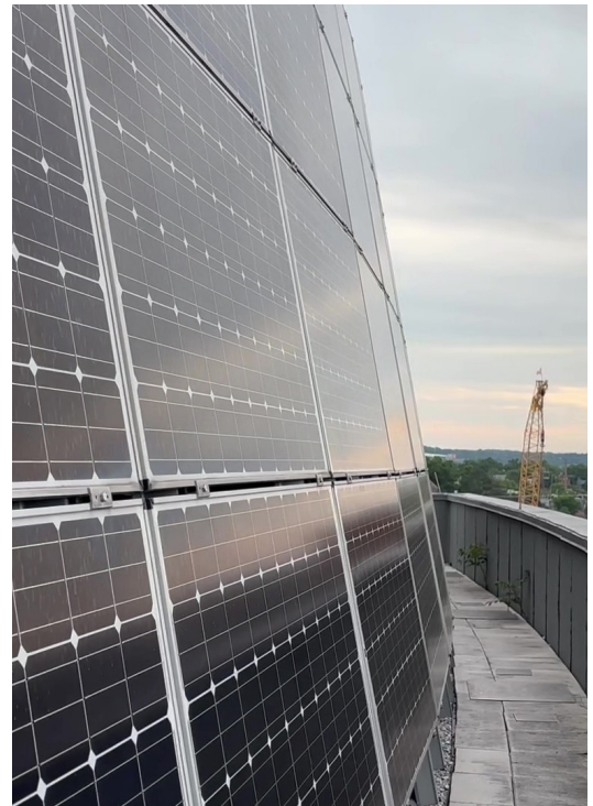
Solar panels on AlexRenew's environmental center.
