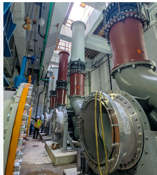
The new pumps and piping are located 60 feet below ground in AlexRenew's massive pumping station.
