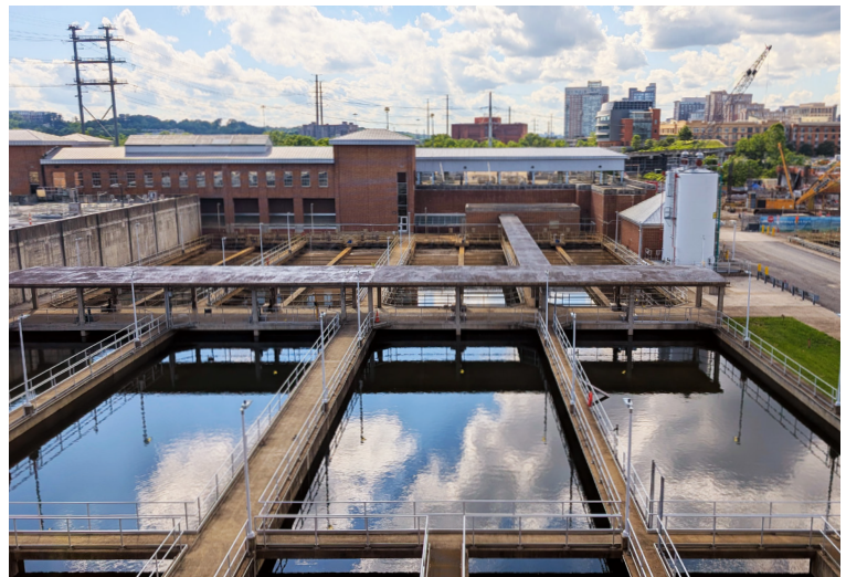
AlexRenew's secondary settling tanks and Biological Reactor Basin.
