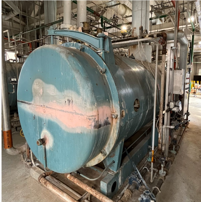
One of five AlexRenew boilers
