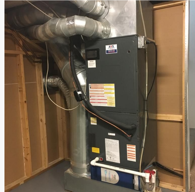
A furnace in a home
