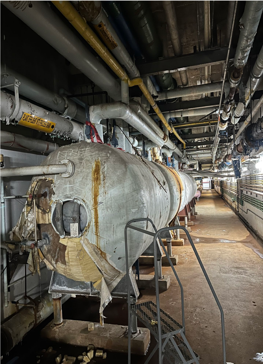
AlexRenew’s Condensate Surge Tanks in Gallery 8
